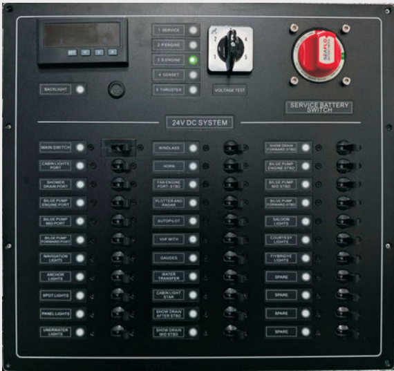
24V DC 1+32 distribution switchboard (unpowered mode)
