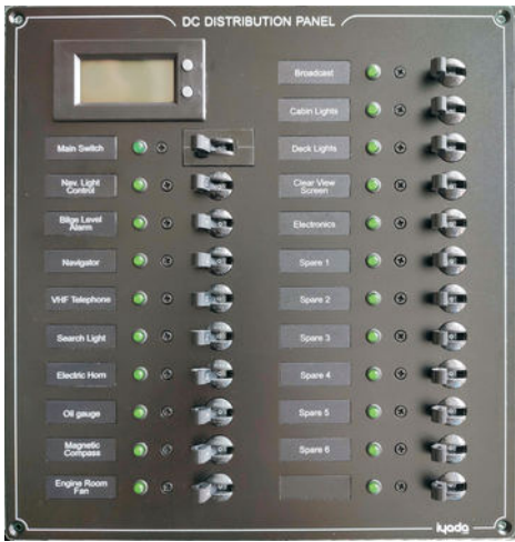
1+21 DC Distribution Switchboard (without backlight)
