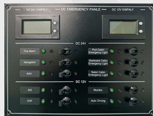
6-channel 24V+4-channel 12V DC emergency power distribution switch combination board
