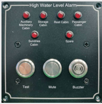
6-channel switching bilge high water level alarm panel
