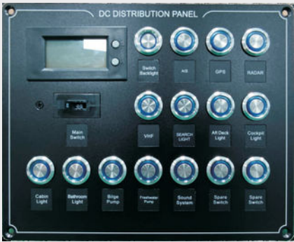
DC 1+15 distribution switchboard
