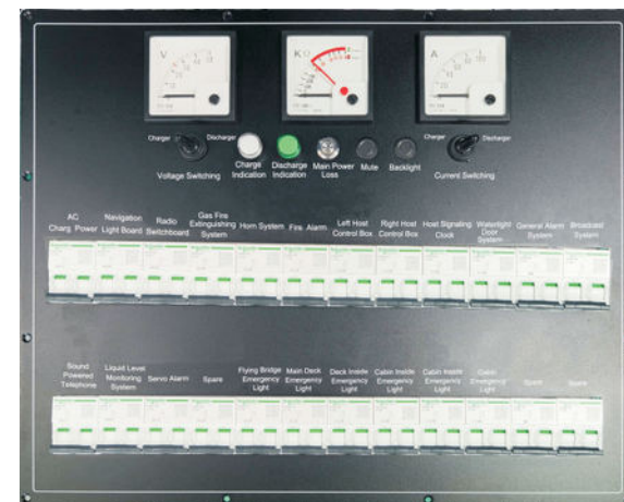
Battery charging/discharging 24-way power distribution control switchboards
