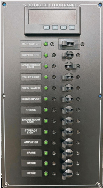
DC-1+12 DC distribution switchboard (backlight off)
