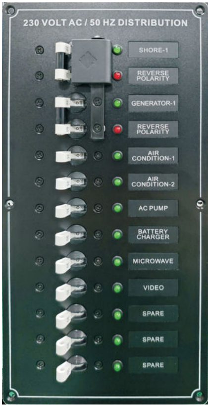
230V50Hz-AC AC-2+9 distribution switchboard
