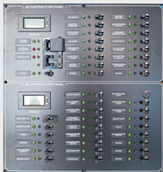
DC 1+22 AC 2+17 Combined Distribution Switchboards
