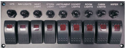
8-1 DC Distribution Switchboard
