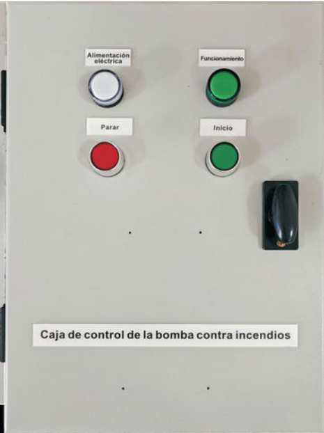
Fire pump control box
