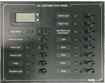
1+13-DC distribution switchboard (without backlight)
